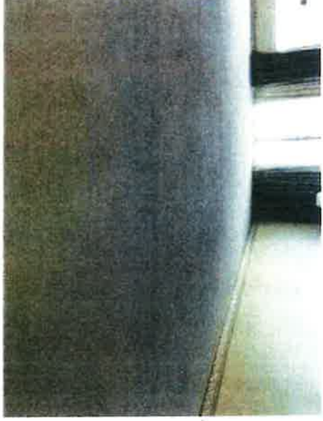
Photo 12: Budget Inn Ceiling Surface Material (HA-06)
