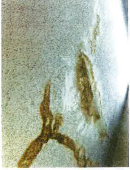
Photo 4: Knights Inn Ceiling Surface Material (HA-04)
