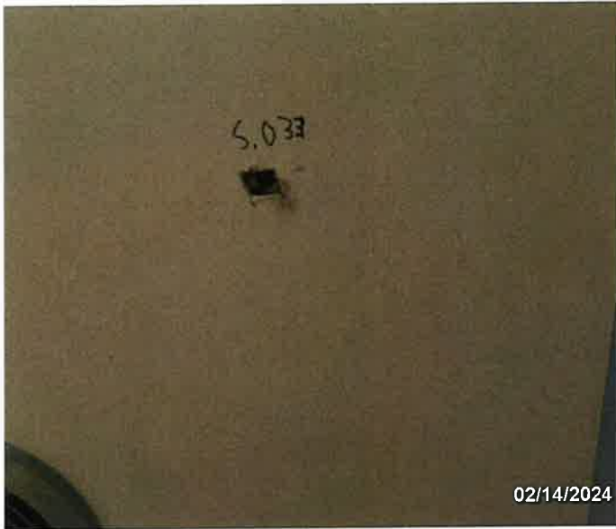
Picture 7. Sample S.033 in Bathroom 1/2 (tub/shower) ceiling board (2% Chrysotile).
