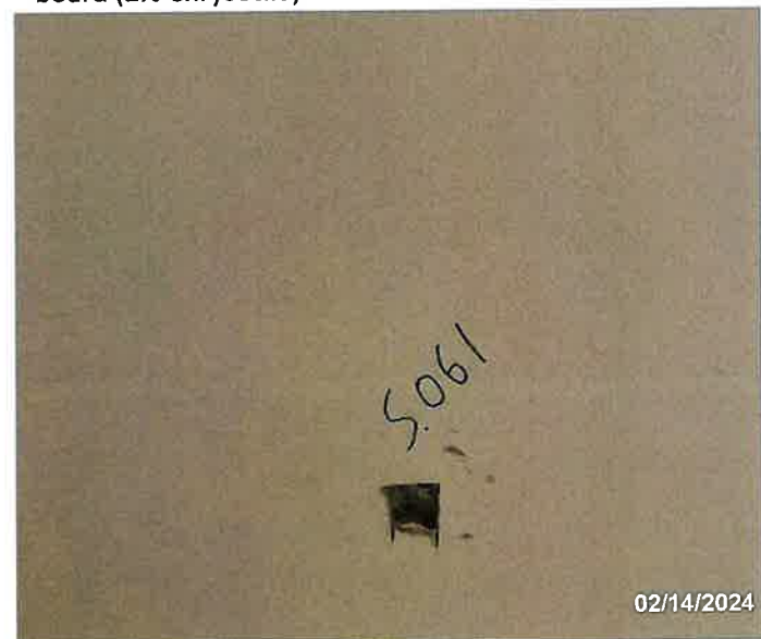
Picture 12. Sample S.061 in the hallway to bedrooms ceiling board (2% Chrysotile).
