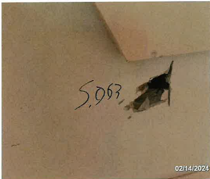
Picture 13. Sample S.063 in the hallway to bedrooms closet wall board (2% Chrysotile).
