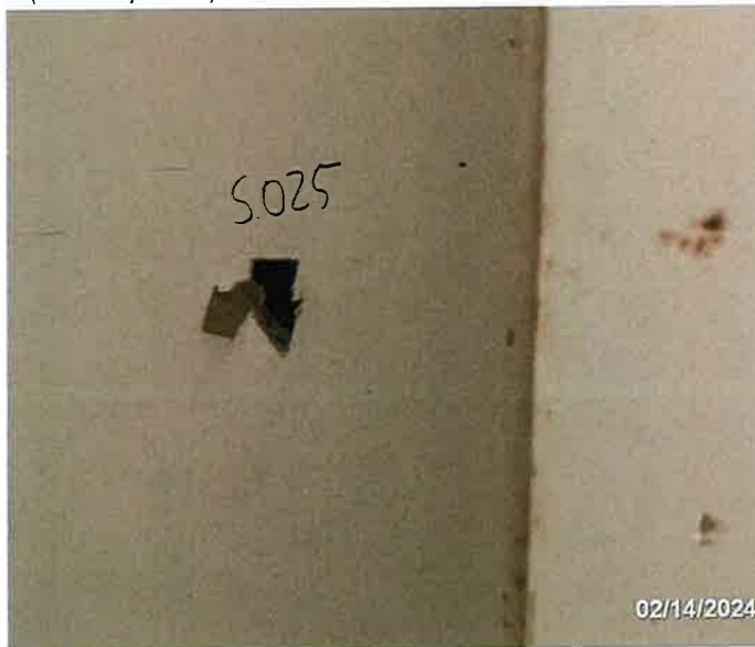
Picture 5. Sample S.025 in Bedroom #2 Closet wall board (2% Chrysotile).
