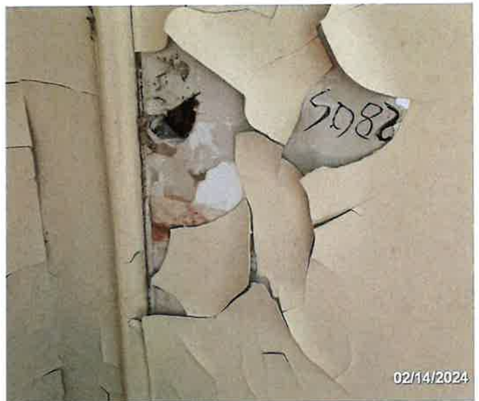
Picture 14. Sample S.082 in Living Room #1 wall board (2% Chrysotile).
