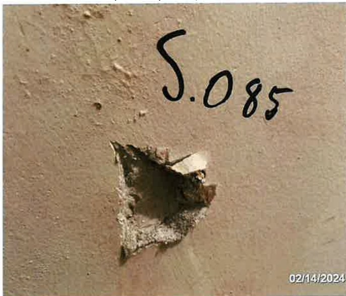
Picture 15. Sample S.085 stairs to safe room wall board (2% Chrysotile).
