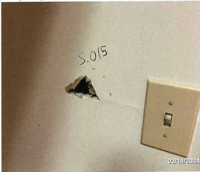
Picture 3. Sample S.015 in Bedroom #3 closet wall board (2% Chrysotile).
