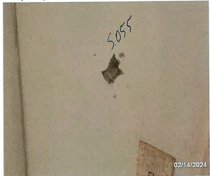
Picture 10. Sample S.055 in Bedroom #1 Closet #2 wall board (2% Chrysotile).
