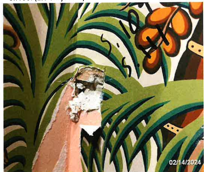
Picture 18. Sample S.111 Bathroom #5 wall board (2% Chrysotile).
