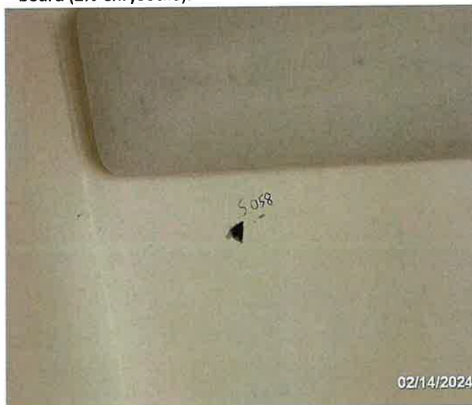
Picture 11. Sample S.058 in Bedroom #1 Closet #2 ceiling board (2% Chrysotile).
