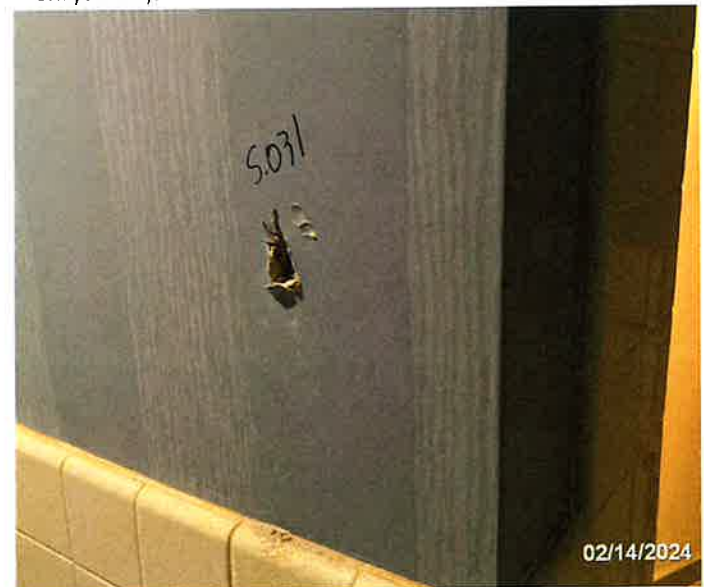
Picture 6. Sample 031 in Bathroom 1/2 (tub/shower) wall board (2% Chrysotile).
