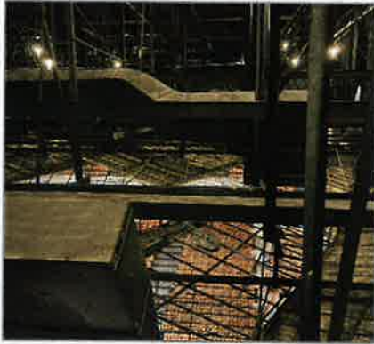
Looking down on main auditorium seating. View of metal structures on mezzanine.
