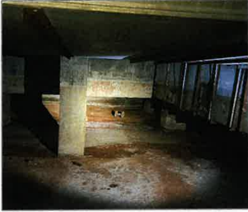
HVAC return duct work below structure and directly below main auditorium hall
