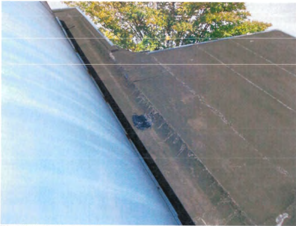
HSA 158-10: Flashing, Sample B.
