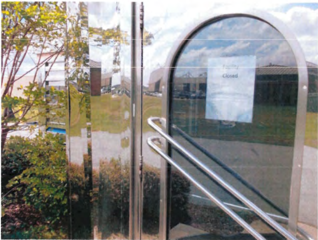
HSA 158-08: Grey Exterior Window and Door Frame Caulk. Sample B.
