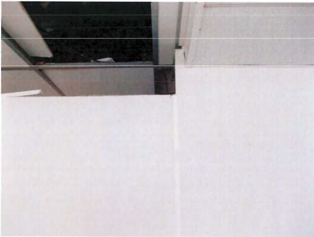
HSA 158-01: Plastic Panel Covered Drywall with Associated Tan Glue. Sample B.
